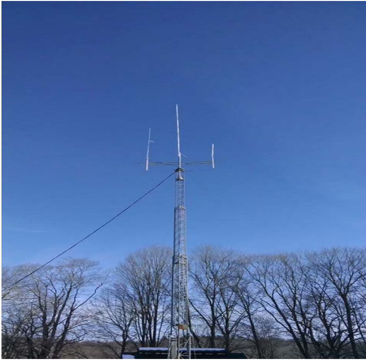
Portable Antenna Setup
