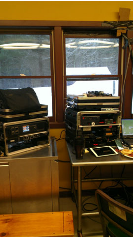
Net Control station (new digital repeater on left.)
